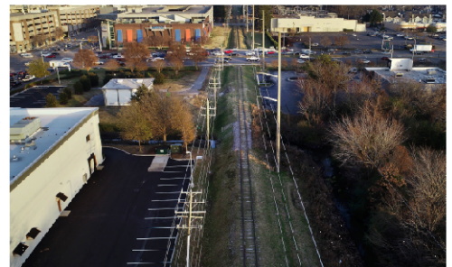
Construction of a segment of the Virginia Beach Trails. The new 10-foot-wide path is located in the heart of the city near the Oceanfront Center.
